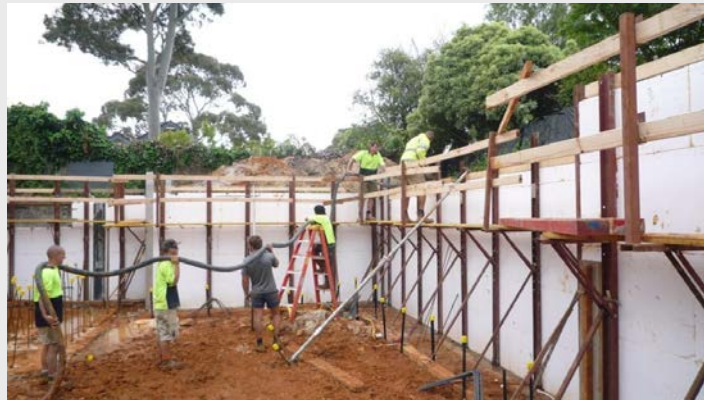
Formcraft team assist with directing line pump for easier control when pouring basement walls, East Brighton
