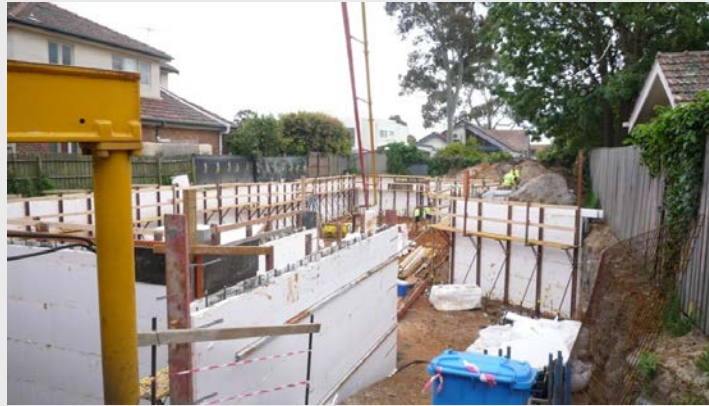
Bracing & safety rails in place, ready to pour basement walls, East Brighton
