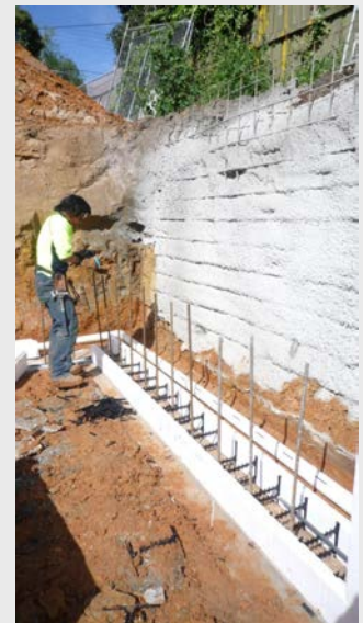
Quang Do setting out first layer of panels into "C" channel, East Brighton
